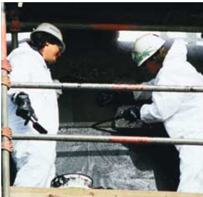
FOAMGLAS® insulation—in 2" (50.8 mm)-thick, 12" x 18" (304.8 mm x 457.2 mm) blocks—being applied to a petroleum storage tank at a West Coast refinery. Industrial applications include pipelines as well as vessels of all types.
