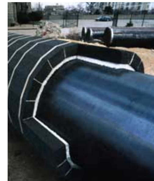
FOAMGLAS® insulation was installed as part of a composite insulation system. It incorporates a one-inch layer of fibrous glass felt material directly around the pipe, covered with FOAMGLAS® insulation.
